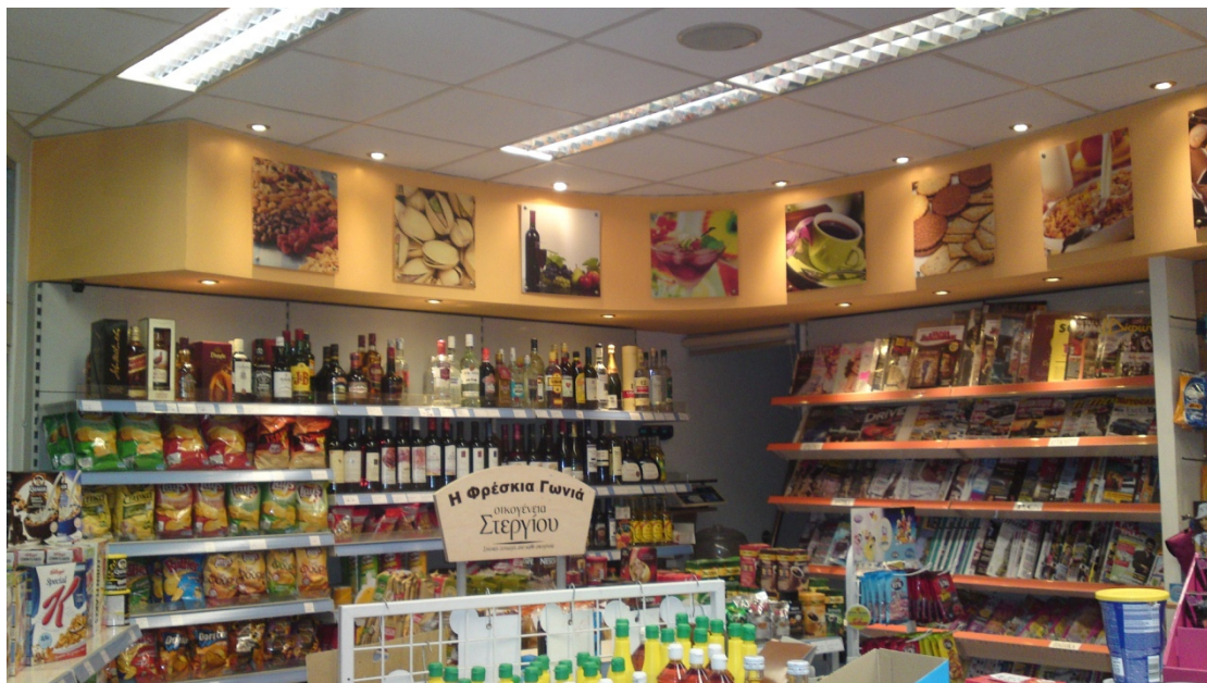
20W LED tube lighting project in Bulgaria
