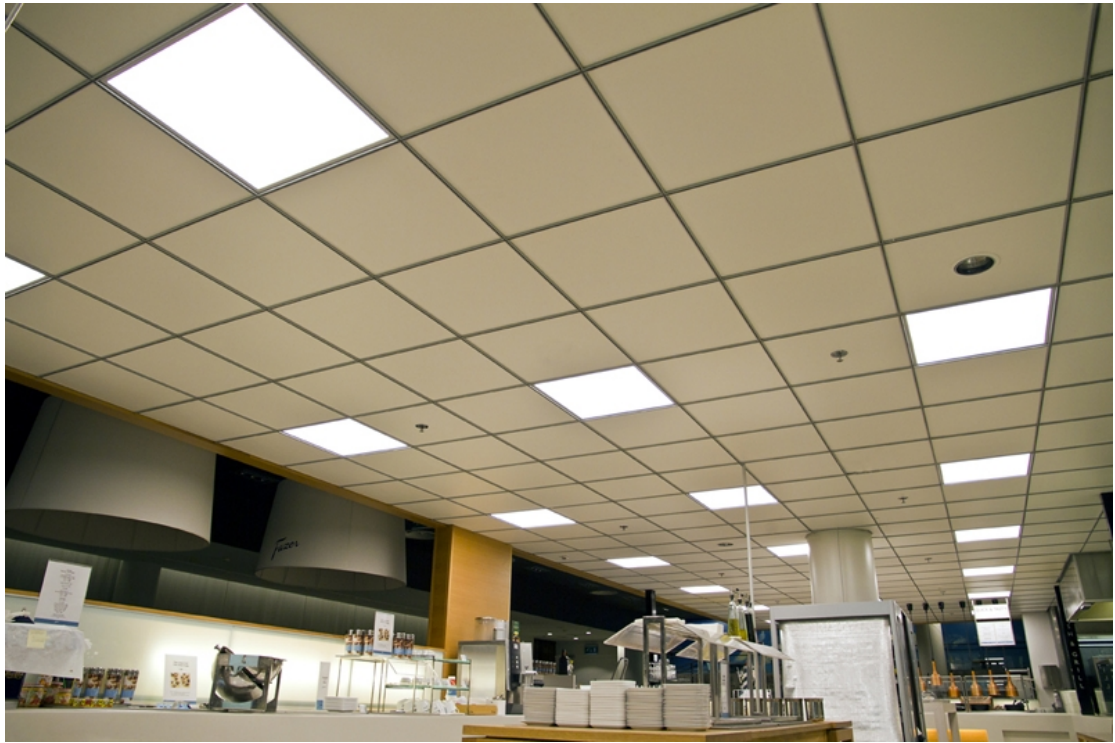
LED Panel Lighting Project in Finland
